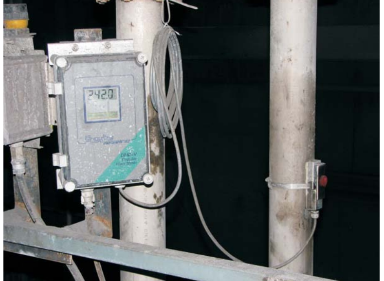
DFM-IV Doppler Flow Meters installed to measure "fly ash slurry" at Xcel Energy's Sherburne County Generating Plant in Becker, Minnesota
