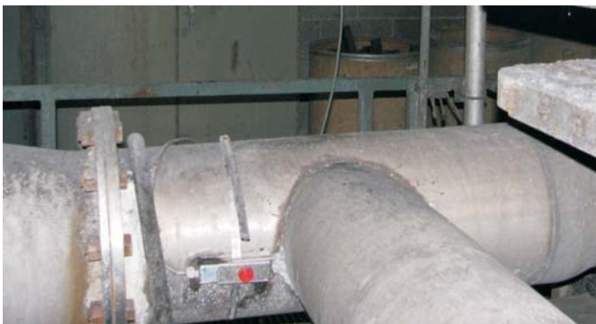
Strap-on ultrasonic sensor is not affected by the abrasive and caustic fly ash slurry
